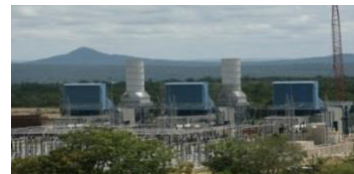
IPP 100-MW GAS TURBINE
