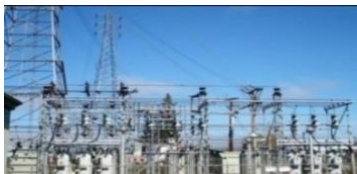
POWER TRANSMISSION GRID
